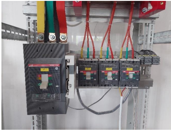
Figure 7. Load-breaker and circuit breakers to consumers
